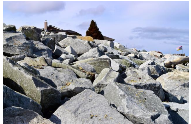
The hardshoring began with Willemar Bluffs. In recent years whole stretches of beach along our coastline have systematically been buried beneath riprap.
