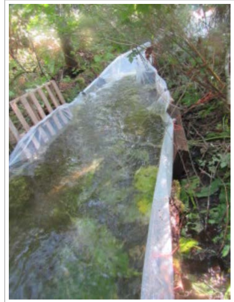
'Slip and slide' used to divert water from the work area. Photo: K. Clouston
