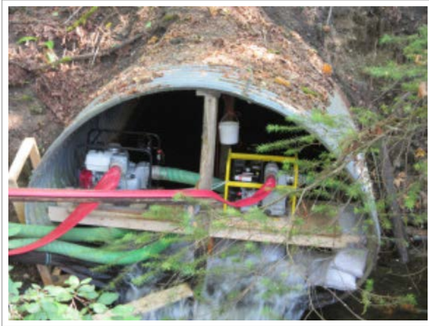
Some of the pumps and hoses for Comox Logging Road culvert improvements. Photo: K. Clouston
